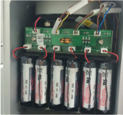
Figure 4-1 Battery placement location
